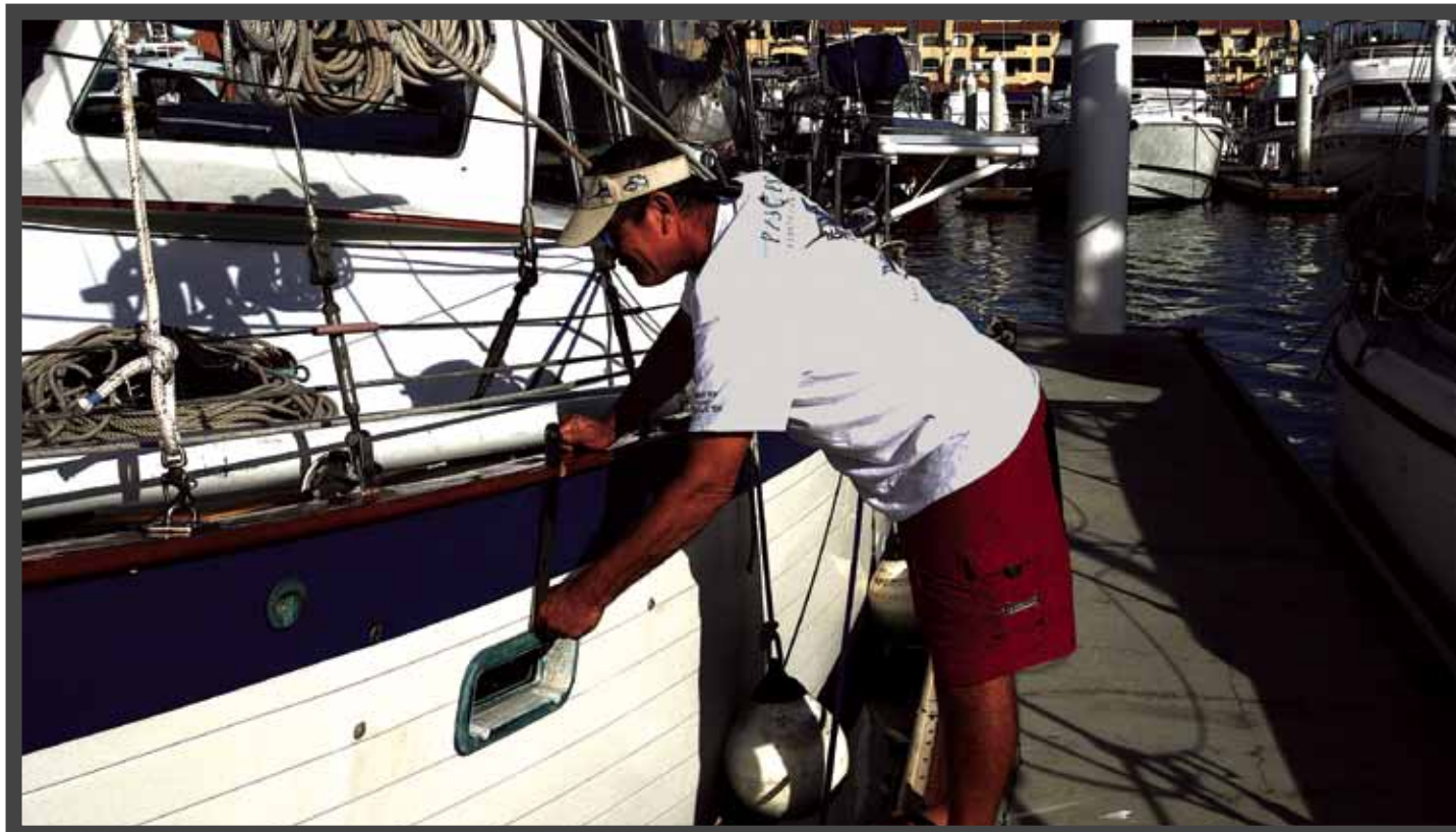
Alex, a local marine worker, fits the newly fabricated chain plate to the outside of the hull of Carricklee.
