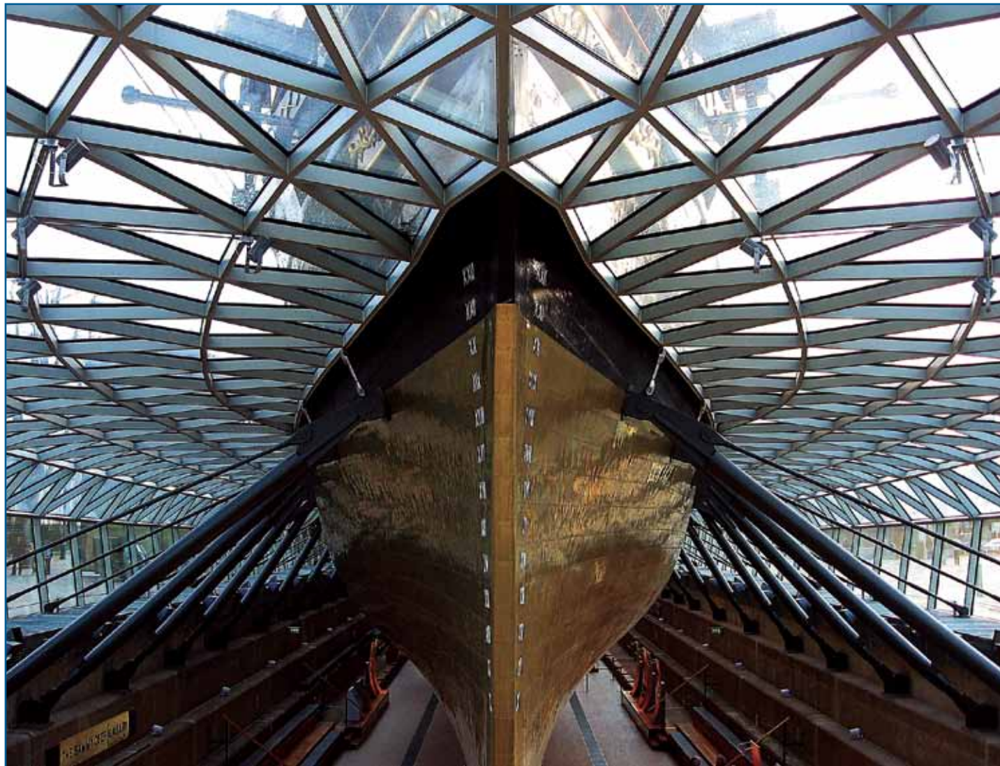
The clipper's hull is held ten feet above the floor of the dock by angled props that tie into the new internal framing. The ship does indeed appear to be "floating" in air!
